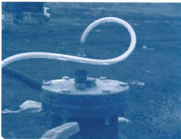
Figure 5.5 Condensate in connection tubing during sampling
