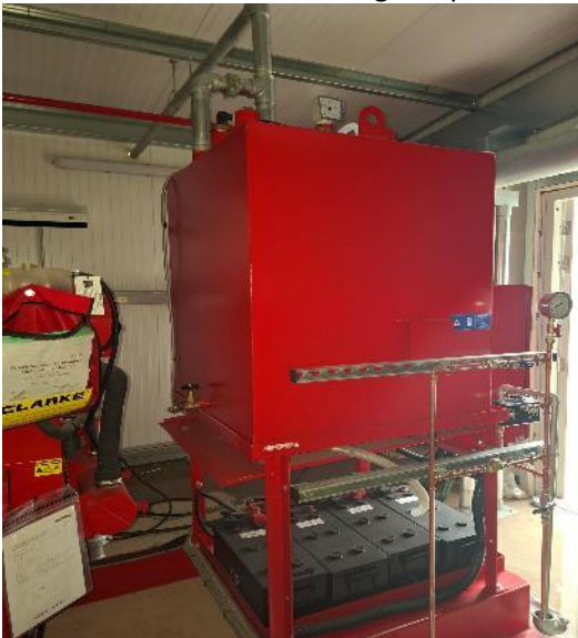
Figure 4: Emergency diesel fire pump fuel tank photograph
