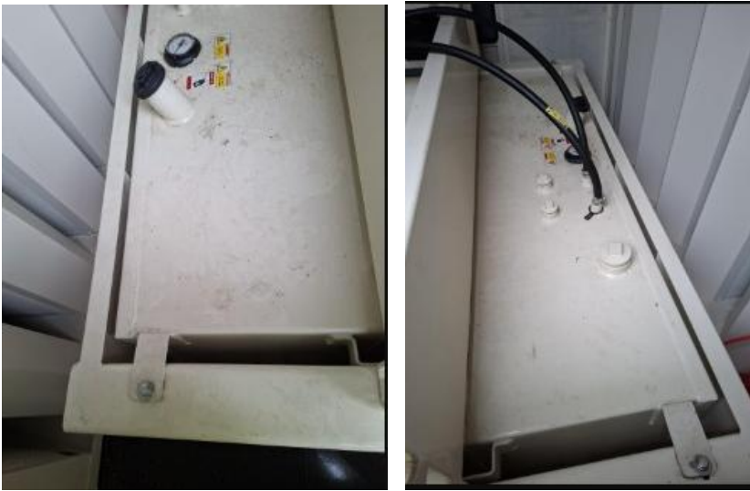
Figure 3: Emergency Diesel Generator fuel oil storage photographs
